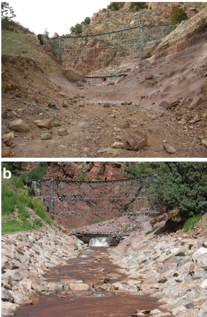
Fig. 7. (a) Paved channel bed and banks extending ~60 m downstream of lower fence, 21 March 2014; (b) Channelized reach downstream of lower fence, 9 August 2014.
